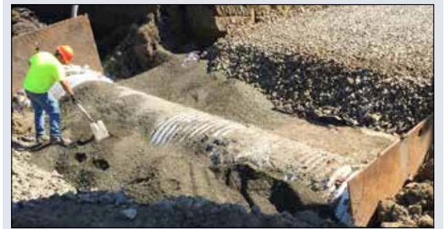
Construction worker spreads gravel over a culvert that runs underneath the Kinsman road extension project.
