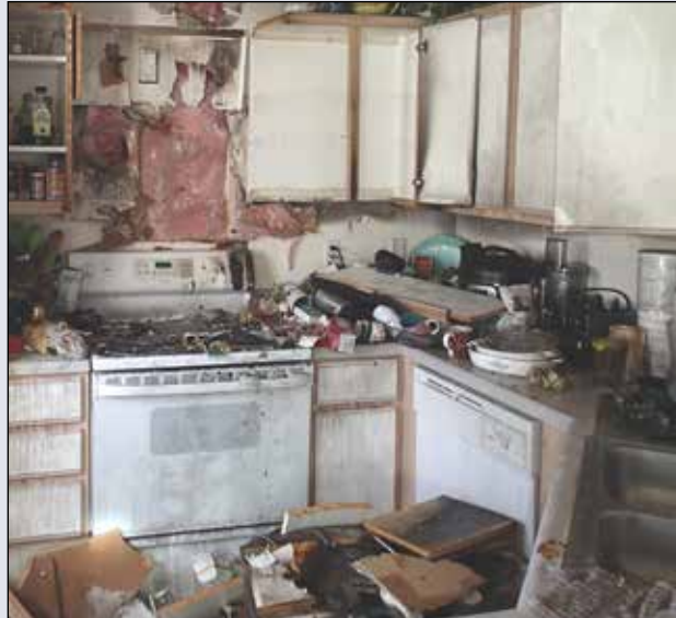
This kitchen fire was caused by unattended cooking at a home in Wilsonville this April.
