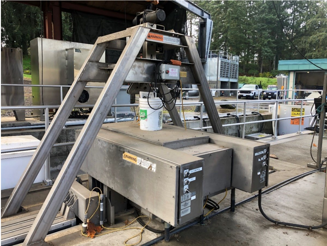
Figure 2-1. Existing TrojanUV4000 system
