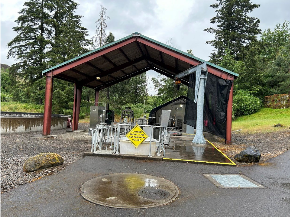
Figure 3-4. Existing Wilsonville WWTP UV disinfection area
