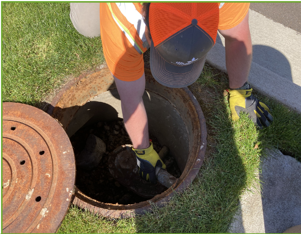
Chad inspecting an Air Release Valve (ARV)
